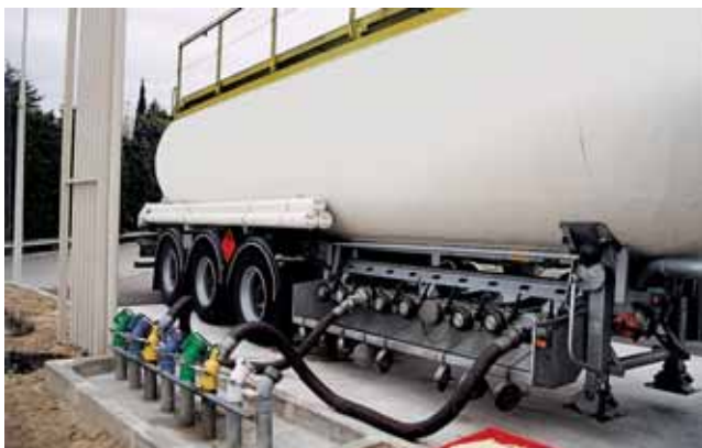
Tank-truck Unloading Equipment
